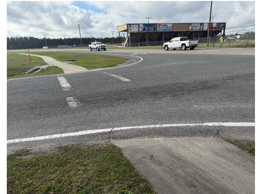
WORN CROSSWALK MARKINGS ON WB APPROACH
