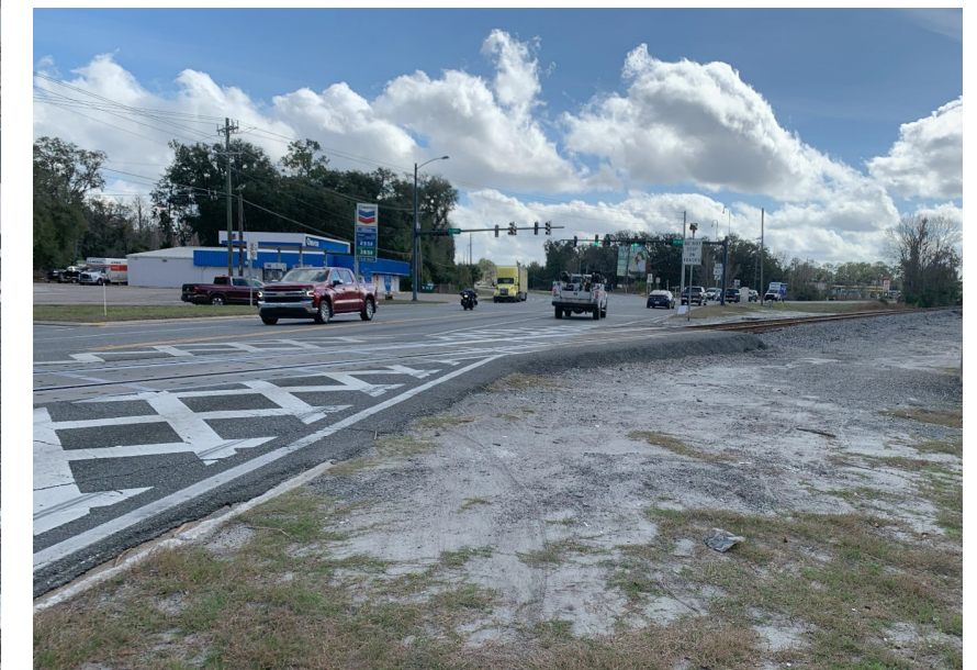
PAVEMENT EXTENDING BEYOND ROADWAY WITH TRAIN TRACKS
