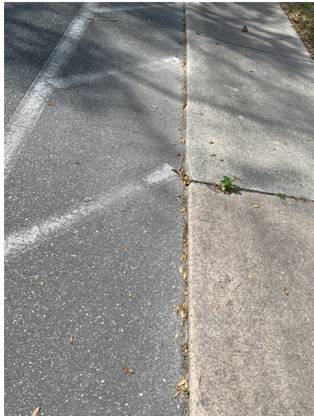
SIDEWALK IS FLUSH WITH ROADWAY AT TIMES
