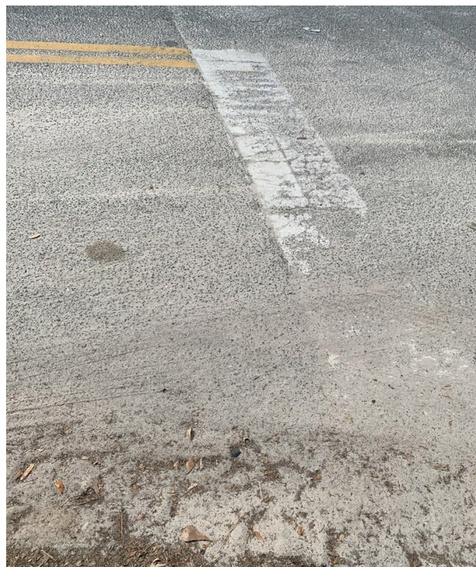
FADED STOP BAR AT SW TUSTENUGGEE AVENUE AND CR 18
