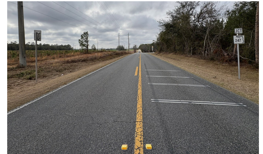
WESTBOUND APPROACH TRANSVERSE RUMBLE STRIPS
