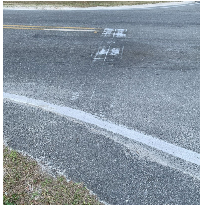
FADED STOP BAR AT SW TUSTENUGGEE AVENUE AND SW HERLONG STREET
