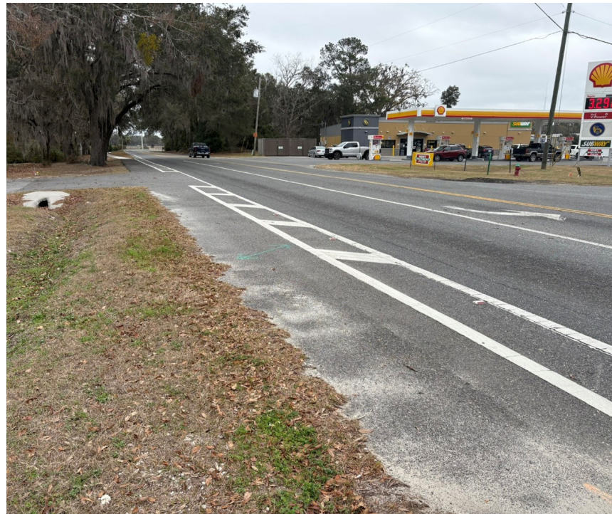
MISSING SECTION OF SIDEWALK
