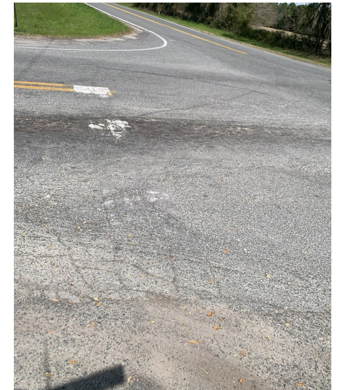
FADED STOP BAR AT INTERSECTION OF SW TUSTENUGGEE AVENUE AND SW CR 240
