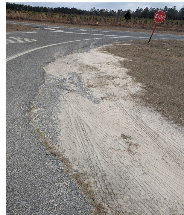
VISIBLE RUTTING FOR EASTBOUND RIGHT
