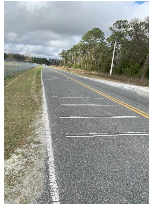
WORN RUMBLE STRIPS ON EB APPROACH
